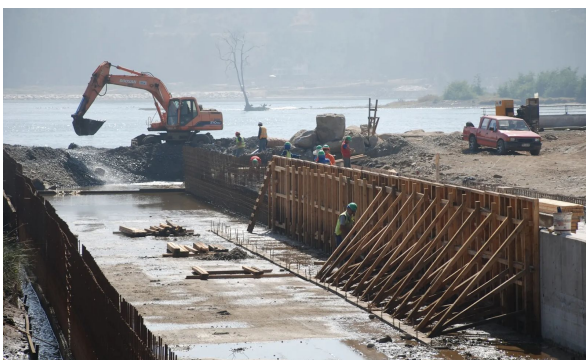
A newly constructed lagoon designed to help flooding after Constitución was damaged by the tsunami.
